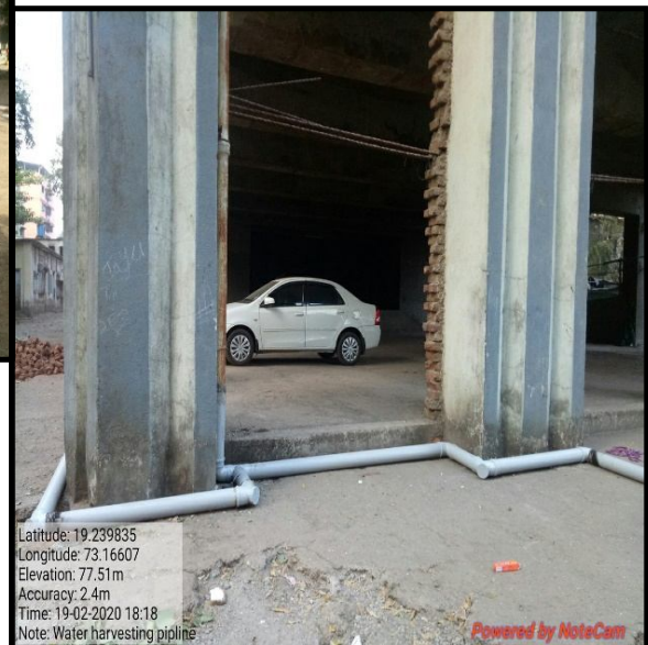
Photo of rain water harvesting pipes
