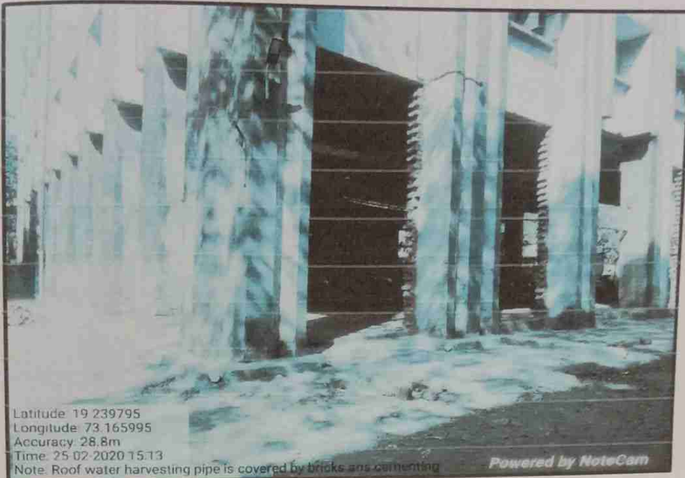
Roof top rain water harvesting pipes is covered by bricks and cementing
