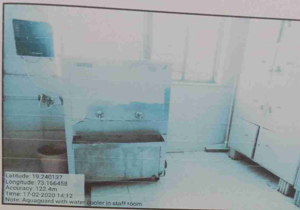
Clean and cool Drinking water facilities provided in the staff room (Aqua guard with water cooler).
