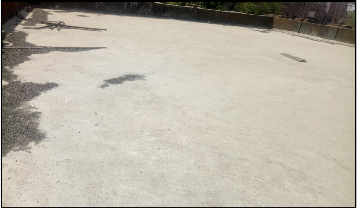
Catchment area of building here roof top rain water harvesting
