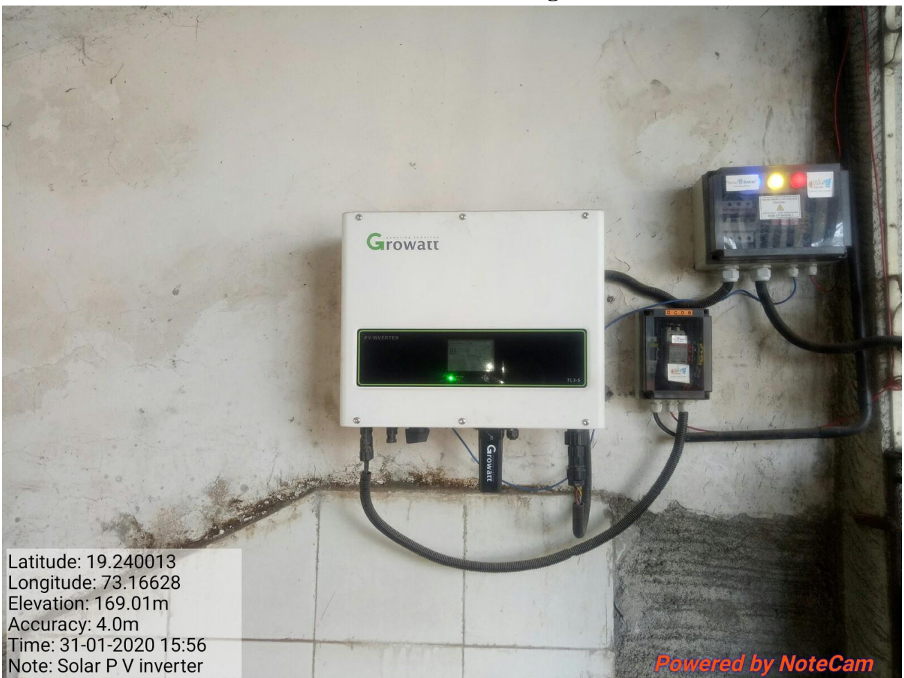
PV inverter of solar
