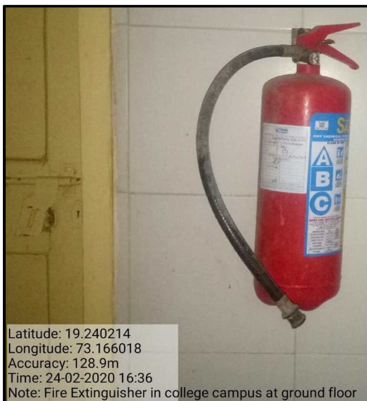
Fire Extinguisher in college on first floor Fire Extinguisher in college on ground floor
