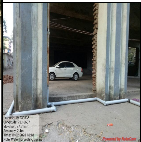
Photo of rain water harvesting pipes
