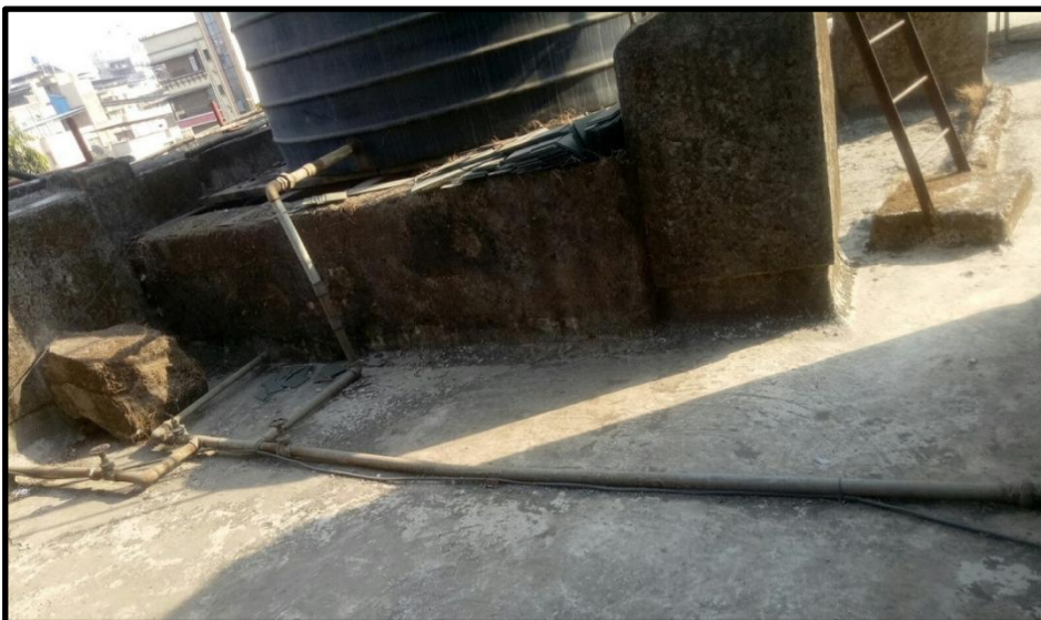
Water storage tank pipeline of water supply to washroom
