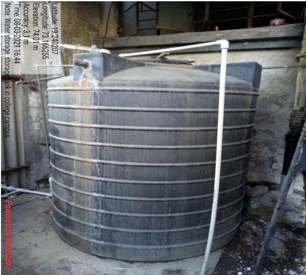
Water storage Tank
