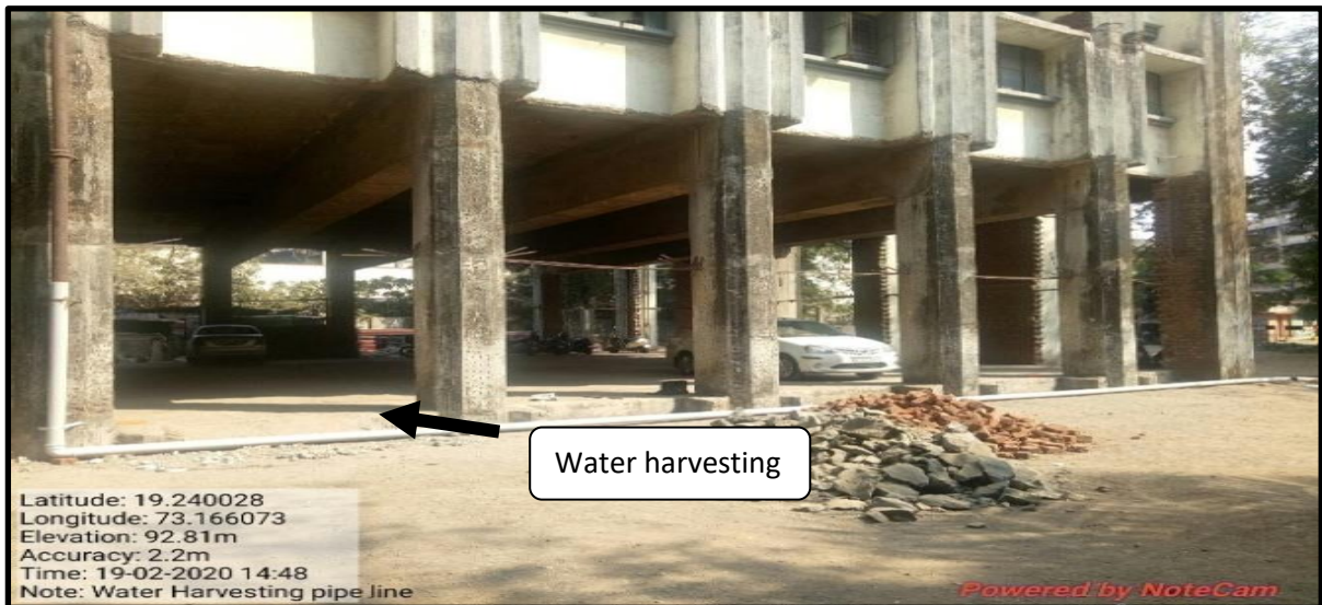
Collection Harvesting water pipeline
