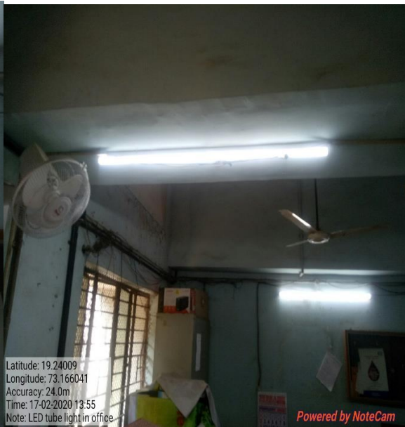
LED Tube light used office
